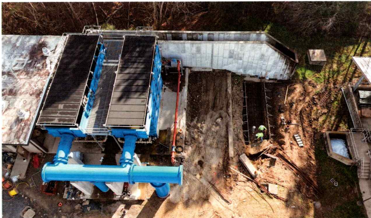
Davidson Drive WWTTP – Filter Pads for Two New Tertiary Filters
